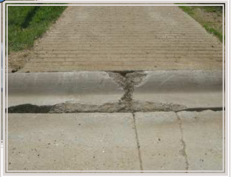
Kerb before repair
