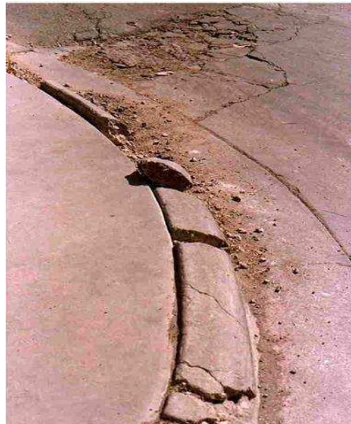
Damaged kerb and road - Before
