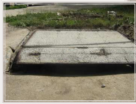
Pit before repair
